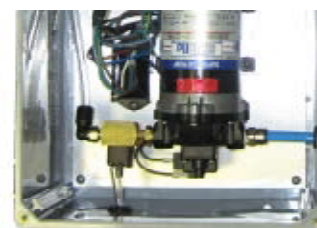
Cabinet outlets configured for four cleaning stations.
